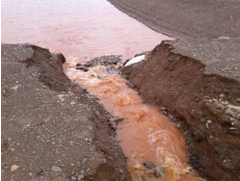
Figure 10. Stronger flow into breach following intervention.
